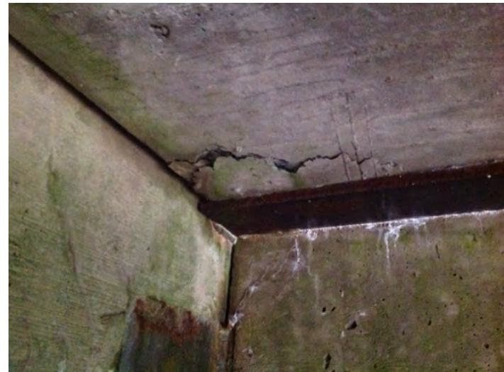
damage to deck panel at downstream right approach
