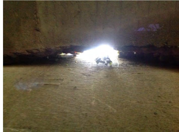
damage to deck panel at downstream left approach
